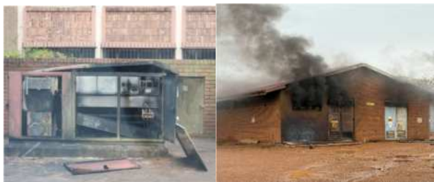
Erasmus Street Substation, Koedoespoort Substation
