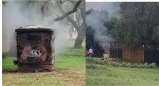
Substation Trevor Street Meyers park/Seema Building in Watermeyer Street
