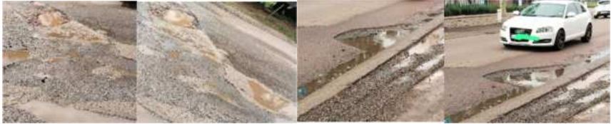
Potholes in Dykor Road next to the Silverton Cemetery
